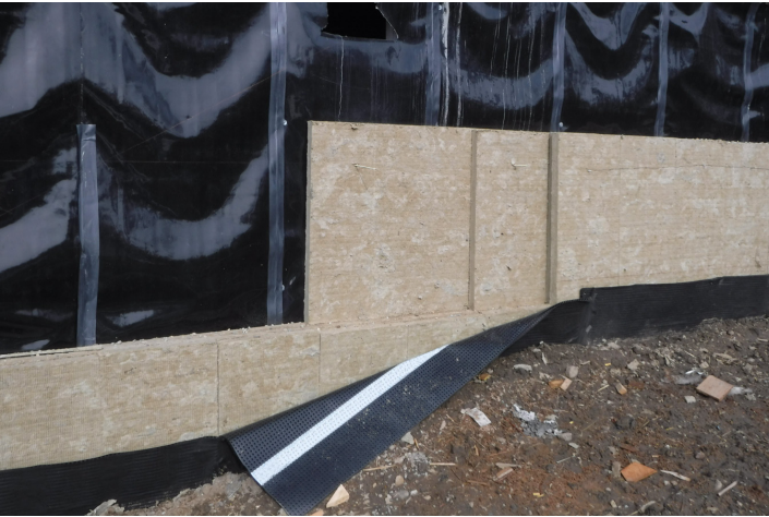
Figure 7: Stone wool insulation used at the transition from above-grade to below-grade enclosures
