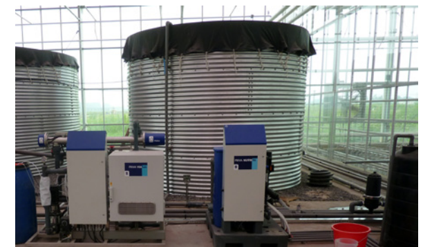
Figure 12. Standard dosing unit for drip irrigation (right) and UV disinfection unit (left).
